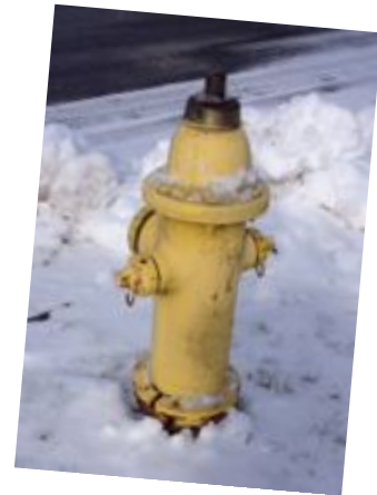
a happy fire hydrant!
